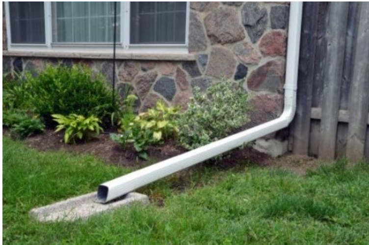
Figure 3.6. A Disconnected Downspout discharging to a pervious area.
