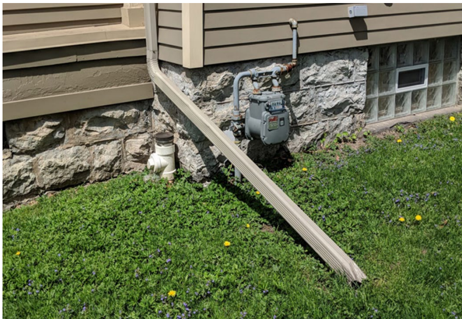
Figure 4.9. Disconnected Downspout (Picture Courtesy Rain Check Buffalo )
