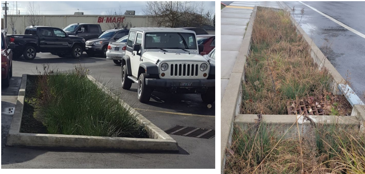
Figure 4.2. A single basin in-ground Stormwater Planter (left), and an in-ground Stormwater Planter with separate cells (right) to allow the water to pond and overflow to each cell down the facility.
